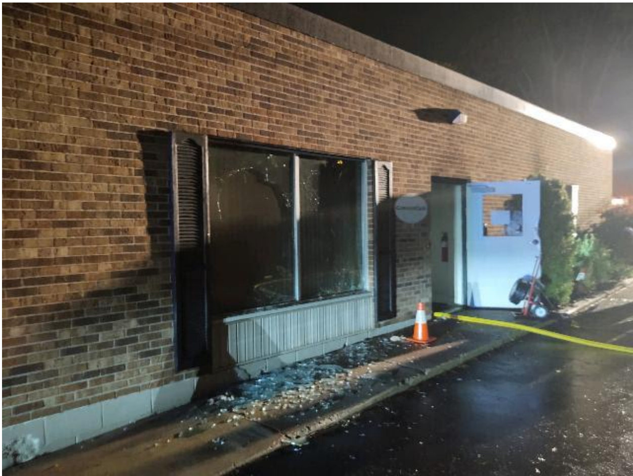
Figure 1. Photo of damage to CompassCare's Amherst facility caused by the June 7, 2022 firebombing.
